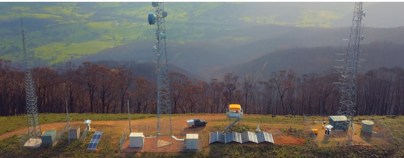
A 5B and Resilient Energy Collective project in Cobargo NSW deployed in 2020. Image courtesy of 5B, an Australian solar pioneer developing prefabricated, pre-wired ground mount technology.
